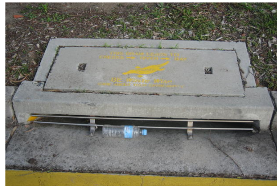
Gutter guards prevent larger littered items from washing into Darebin Creek.
